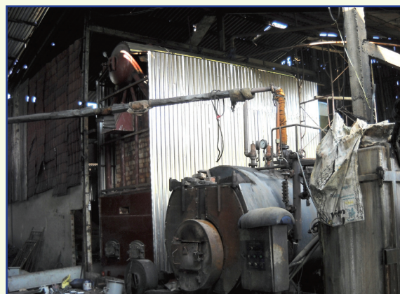
Old boiler using coal and new one using husk with investment of 1,6 billion VND reducing 100% CO 2 emission.
