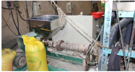
Poor insulation of equipment in a plastic company before CP-RE
