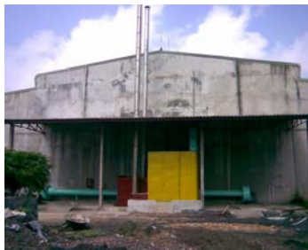
Hot air supply system before CP: 1 high efficient heater
