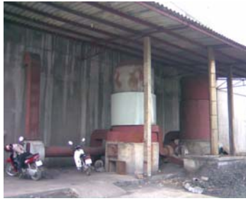
Hot air supply system before CP: 2 low efficient heaters
